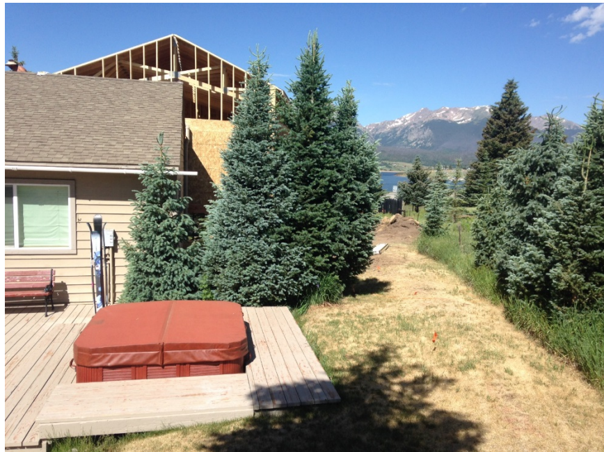
Existing hot tub partially in utility easement.
